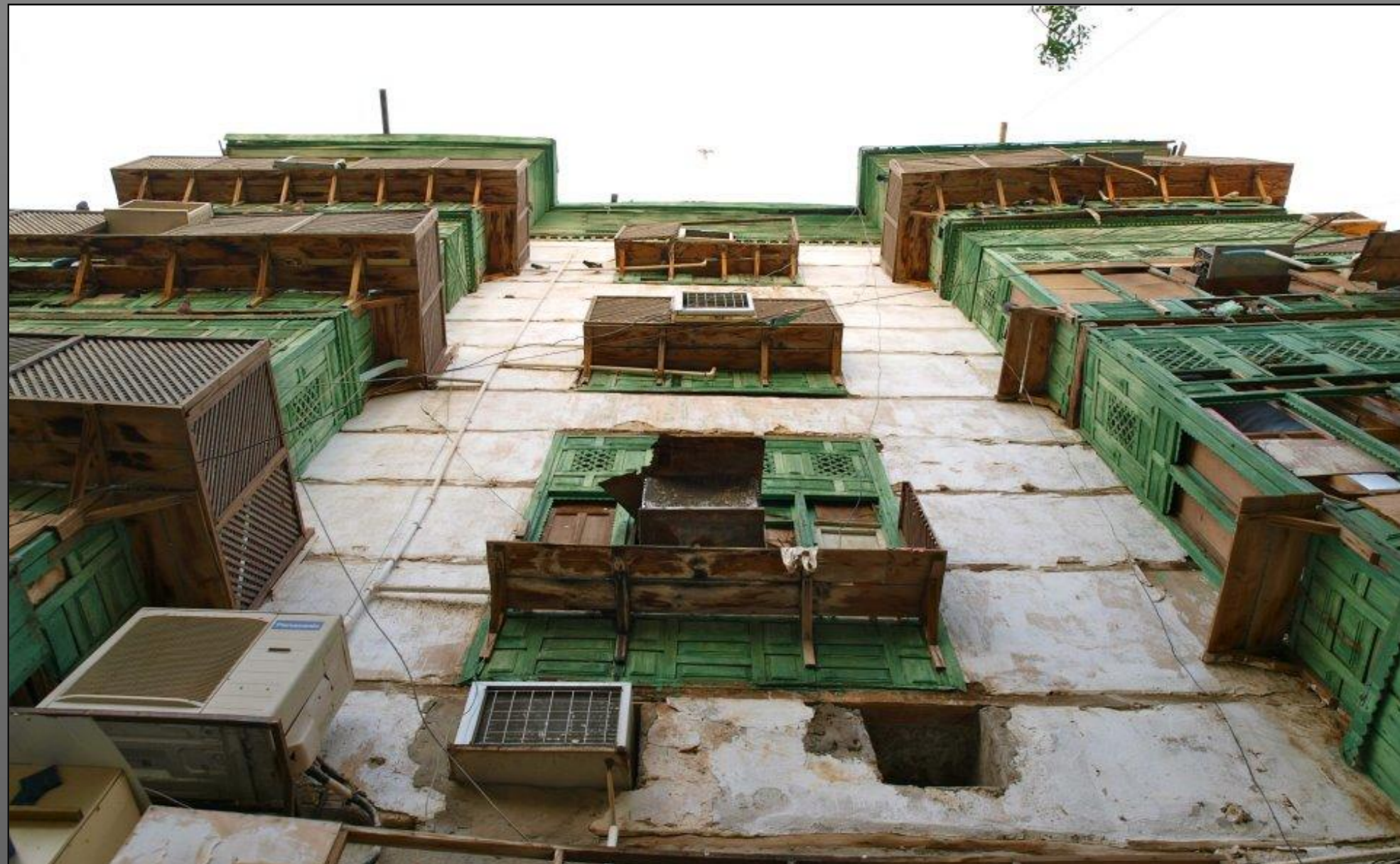
These two photographs show the recent condition of the built environment in the historic core of Jeddah buildings (deterioration) (The Author, 2011)
